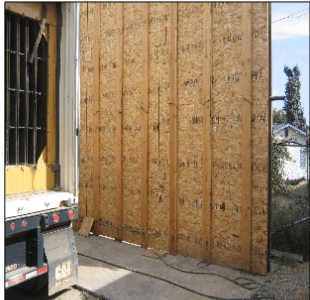
At this location, the project contractor installed a temporary noise barrier to reduce noise pollution at the adjacent residential uses.
