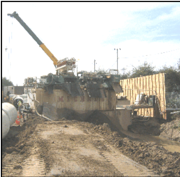
Noise level data was collected for each noise generating piece of tunneling equipment including this soil separation unit.
